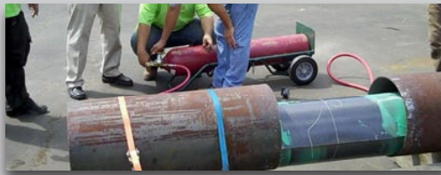
And positioned in the repair area with the aid of a CCTV camera
