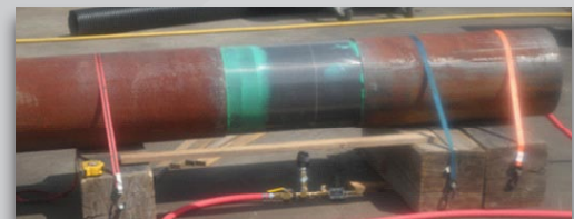
The repaired pipe after installation of a 3-layer thick PipeMedic™ PC26.16 Carbon Laminate, is capable of resisting more than 500 psi (35 bar).
