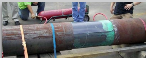
Until it reaches nearly the same 16 inch (400mm) diameter of the pipe
